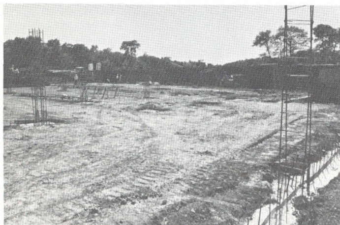
IFDC Phase A buildings come out of the ground. View taken looking southwest in the management area basement. Underground parking area is in right center of picture. Headhouse basement shown in rear center of picture. Outreach/training and main lab wings to be above ground at right center of picture. The construction work continues.
