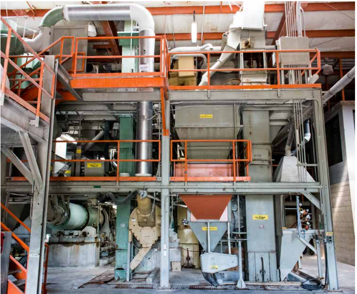
▲ IFDC Large-Scale Pilot Plant
