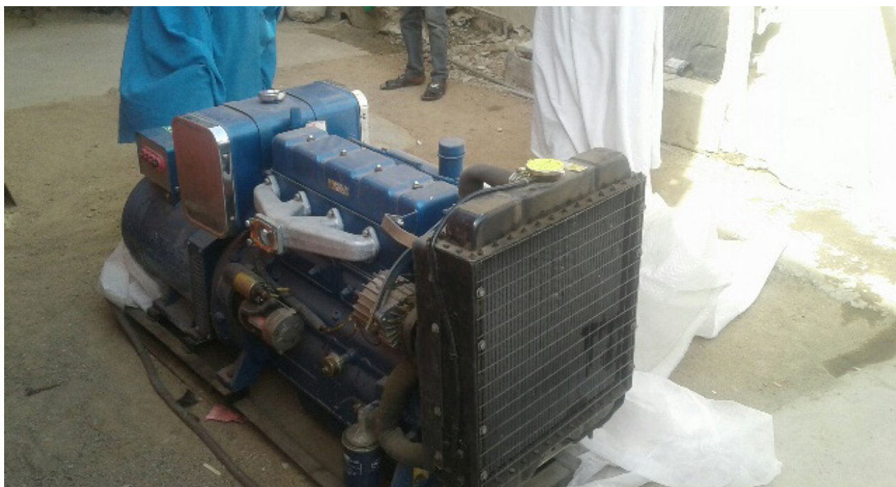
Electricity generator – a fixed asset acquired by a women's cooperative in Kano State; photo by Yusuf Haliru & Associates
