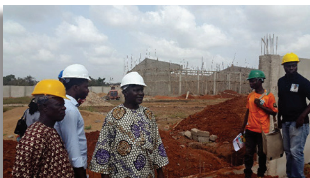
PEA Actors and Town Hall Officials Viewing Construction of the 1000-ton Maize Warehouse in Kétou
